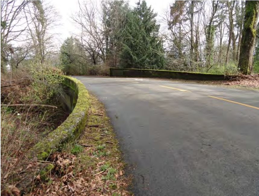
Photo 16. WA_KingCounty_LakeWashingtonBoulevard_0016. Colman Park Overpass No. 2 (contributing resource no. 5) carries Lake Washington Boulevard over Colman Park walking paths, view east.
