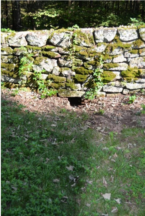
Detail of the stone wall along the Long Lane Approach Drive with a drainage outlet designed at the base to manage stormwater flow.
