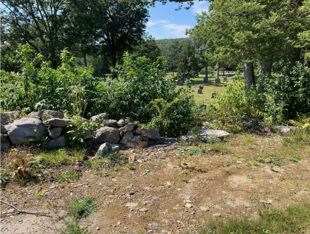
Overgrown staircase and walls near overlook.
