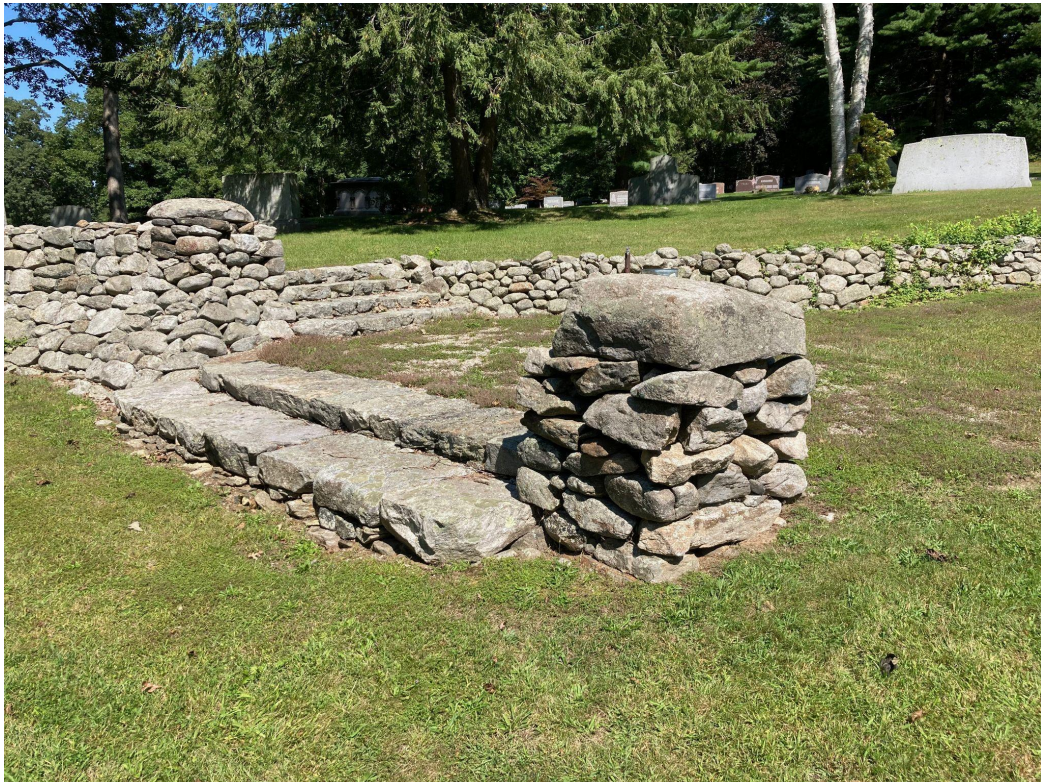
View north to rustic steps incorporated into retaining wall with turf landing, part of wall wrapping valley.
