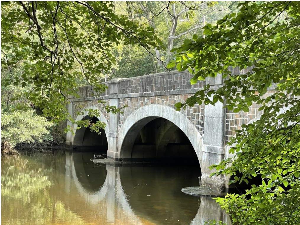
View of the underside of a picturesque bridge over the Mill River.
